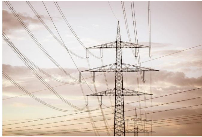
an electricity pylon
